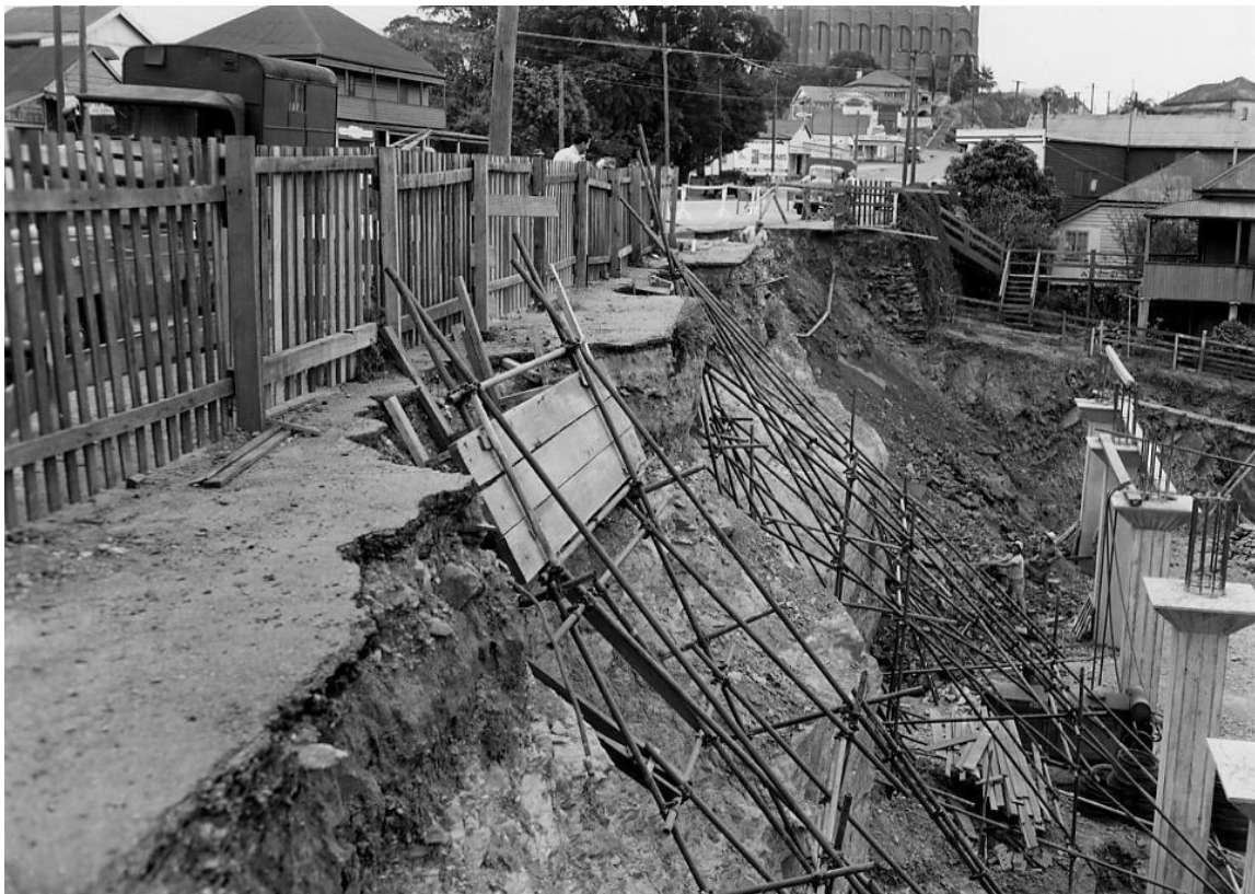
Footpath collapse during construction of the foundations for the Queensland Egg Marketing Board building in 1956 (Brisbane City Archives)
