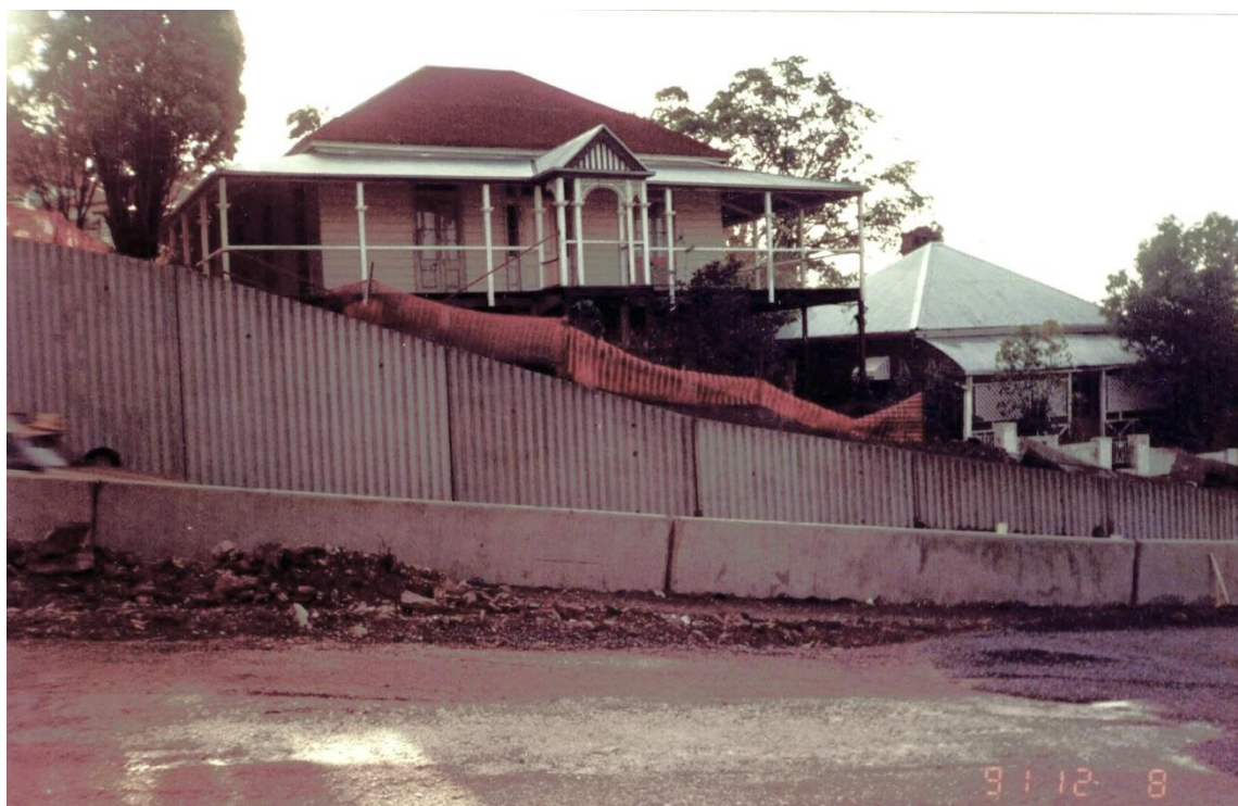
1991 view of Nos 13 and 15 Clyde Street from Hale Street during construction of the Inner City Bypass (BHG Research Library)
